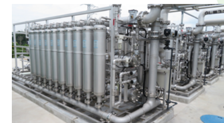
GL module units installed at Kurashiki Plant
